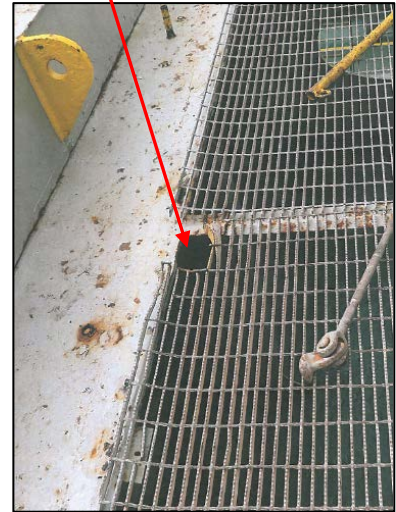
Hole on grating platform 格柵中有孔洞
