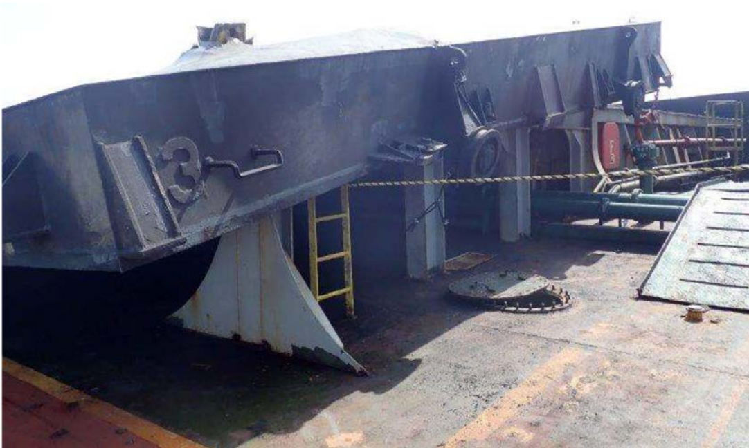
Figure 4 Aft end of No.3 C/H hatch cover port panel
