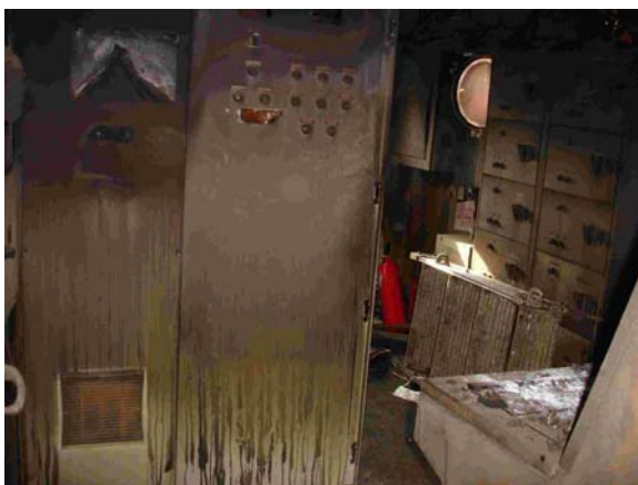
Fig. 19: Cargo Control Room
