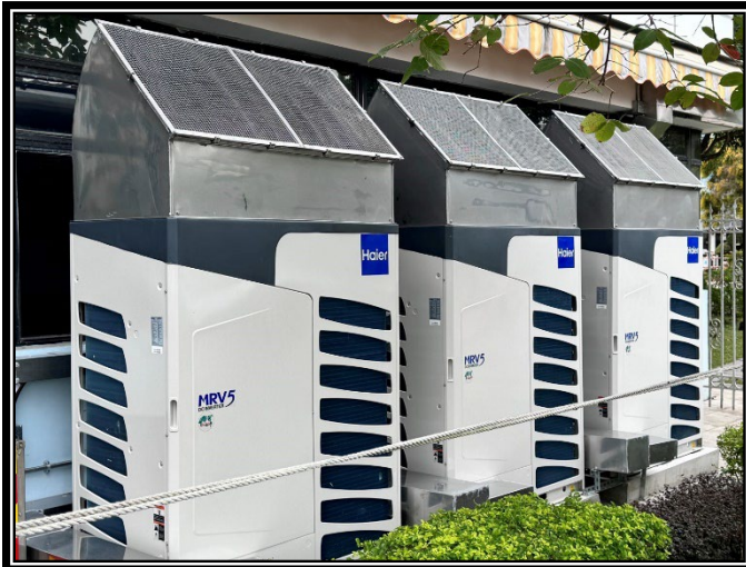
VRV system with VSD Units
