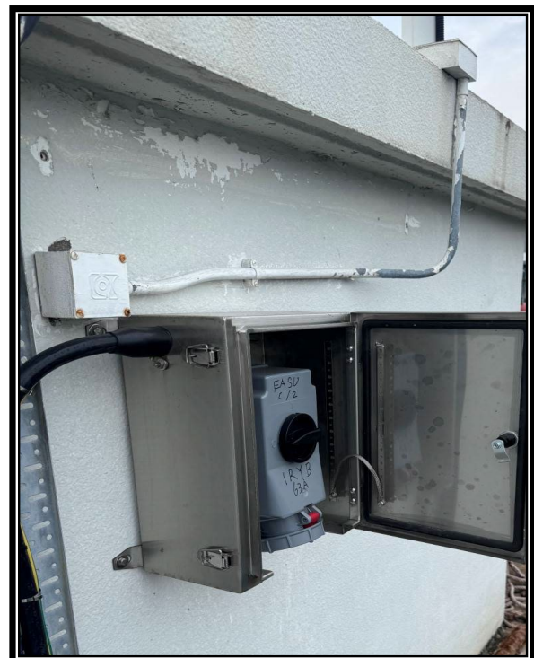
Newly installed 63A 3-phase shore power supply
