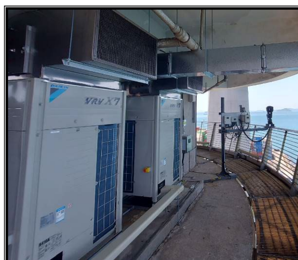
AC project at Kwai Chung Marine Traffic Control Station (KCCS)
