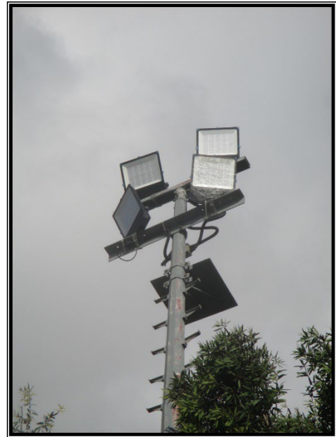
Energy-efficient LED Lights in Western District PCWA
