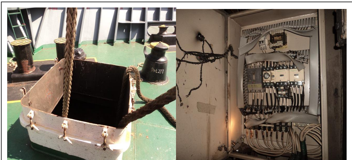
Fig.2 Left - the escape hatch cover blown away. Right - electric control panels deformed and burnt
