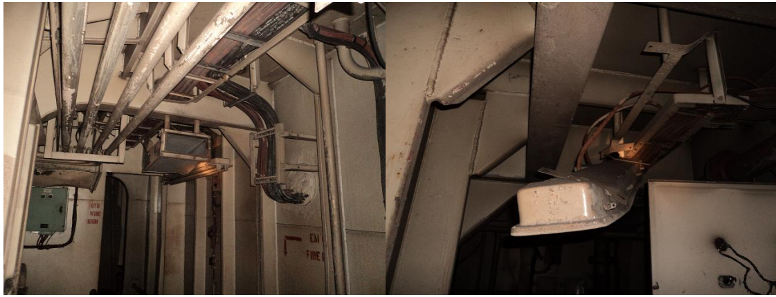
Fig. 3 - Left – 90% of electric cable burnt. Right – all lights broken and damaged
