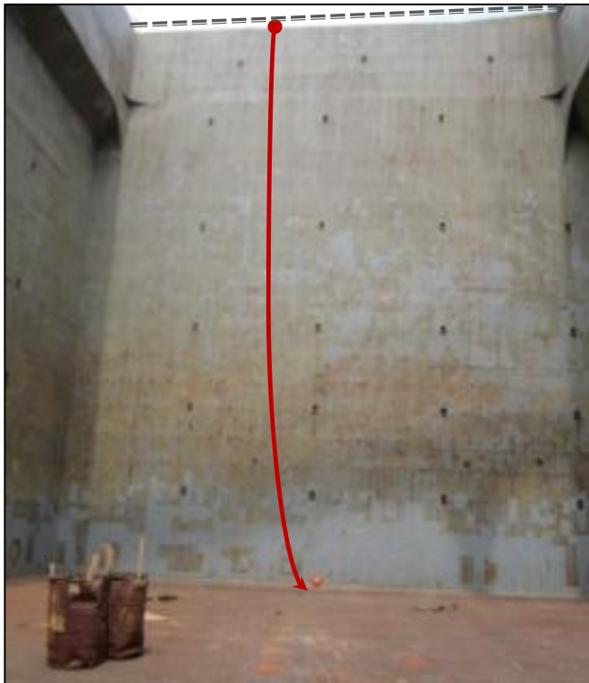
Fig.3 – Cargo hold No.4, the red arrow indicating the fall of AB1.
