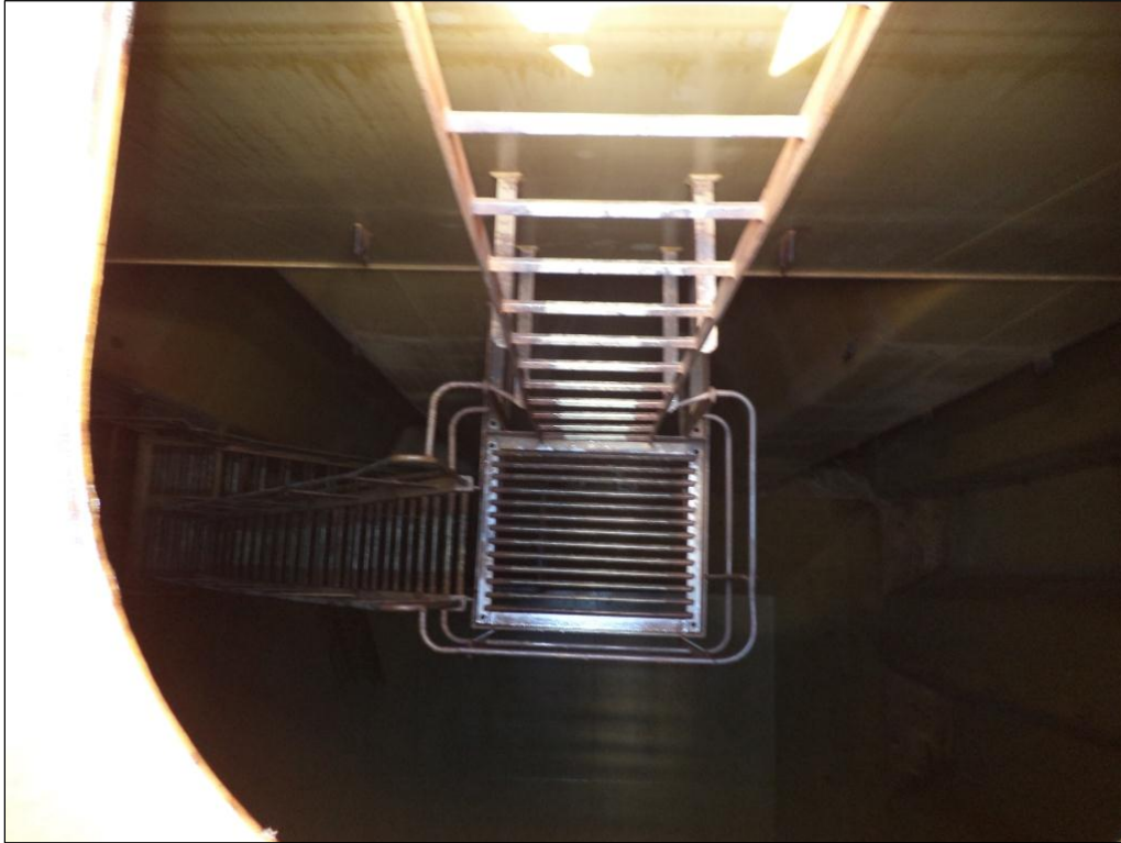
Fig.2 – Access ladder inside 4S COT
