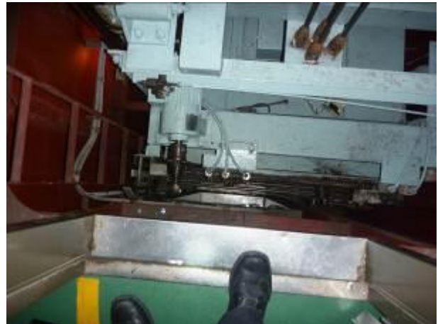
View showing the gap between the cage and bulkhead
