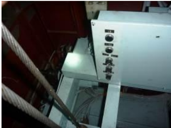
Front view of the control panel
