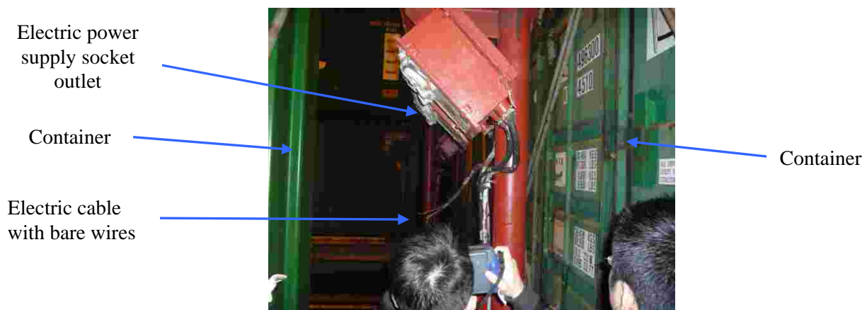
Fig.10: The Electric Cable with Bare Wires at the Walkway
