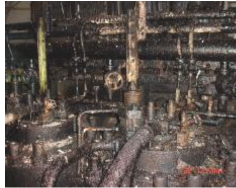
Fig 9: Top of main engine coated with heavy fuel oil.
