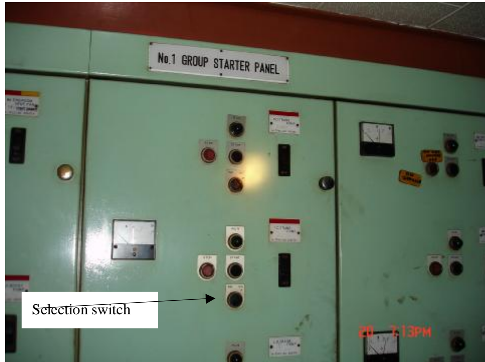
Fig 3: Starter panel for fuel oil transfer pump.
