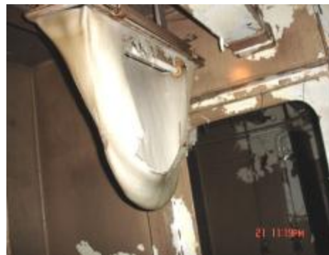
Fig. 16: The light cover was melted by the intense heat.
