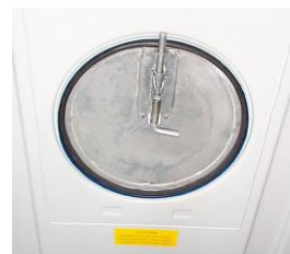
Figure 9.11 Roof hatch internal lock
