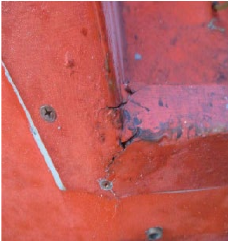
Cracks found in door frame of rescue boat
