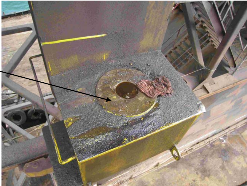
Fig.18: Lower Structure for Supporting the Arm and Hydraulic Support Frame of No.2 Dock Arm
