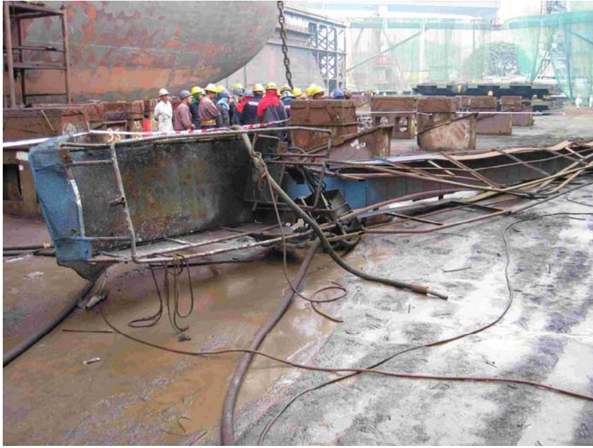
Fig.9: Distorted Platform and Arm Lying at the Bottom of Floating Dock “United”
