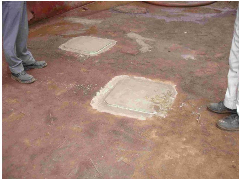
Fig.23: Two Holes were Repaired by Doublers on the Bottom Plate of Floating Dock “ United ”
