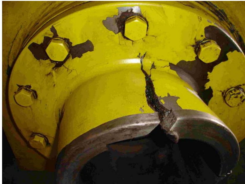
Fig.21: Deformed Upper Coupling with Keyway being Torn Apart
