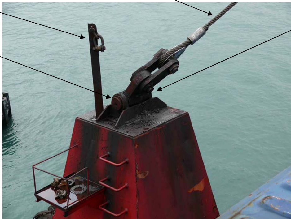
Fig. 3: Top of Anchor Block of Slewing Guy on "Smart Hill No.1"
