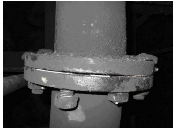
Figure 5: The cut away bolts
