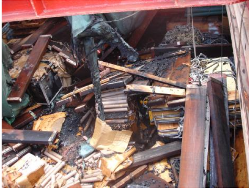
Fig. 5a: Condition of the cargo hold after the fire and the explosion
