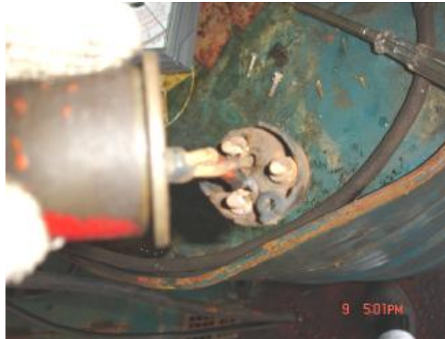
Fig. 5: No earthing line connected to the power plug.
