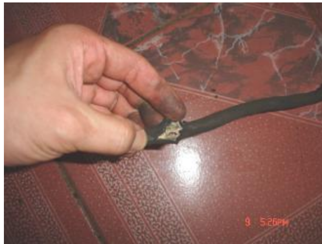
Fig. 4: One of the cleavages of the cable.
