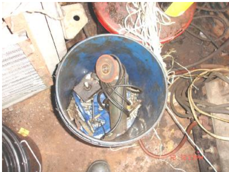
Fig. 3: Portable electrical equipment that required electrical power from the extension power cable
