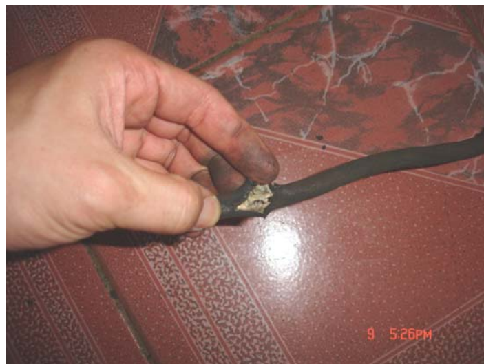
Fig. 2: One of the cleavages of the cable.
