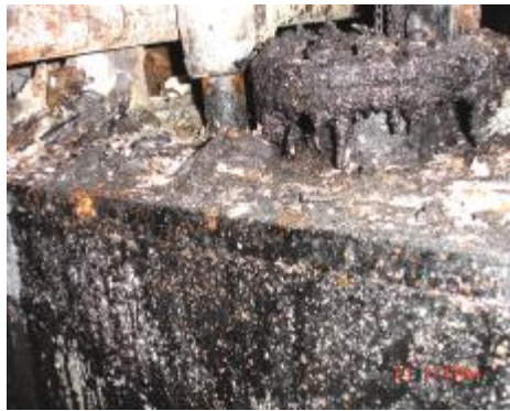
Fig 8: Sign of fuel oil leakage from the top of the boiler fuel oil
