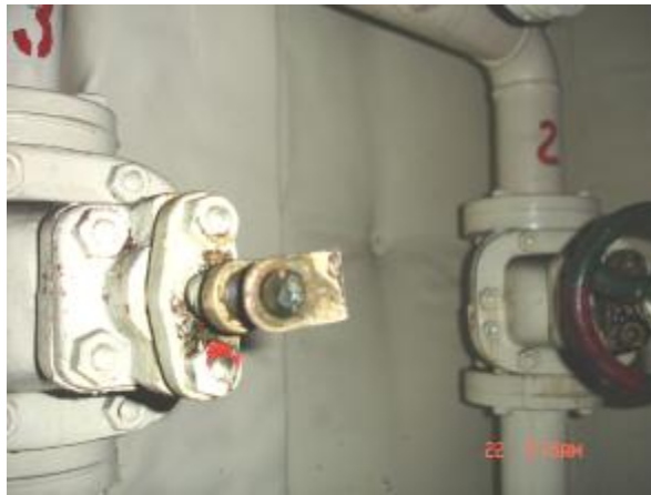
Fig. 23: The valve for the injection of foam liquid to the boiler space was broken during operation.
