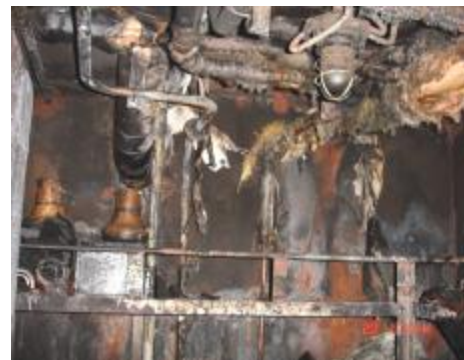
Fig. 18: Equipment in the safety locker were damaged.
