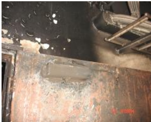
Fig. 19: The connections of the door self closing device was detached.
