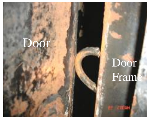
Fig. 20: The ring obstructed the closure of the door.
