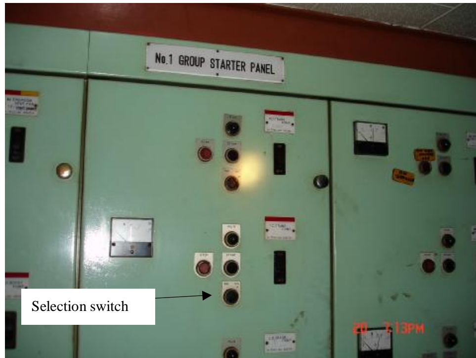
Fig 3: Starter panel for fuel oil transfer pump.
