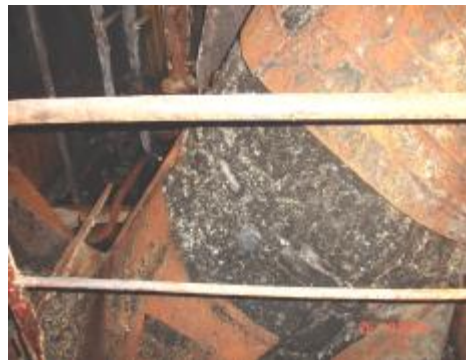
Fig.12: Metal shielding for exhaust M/E exhaust truck deformed and detached.
