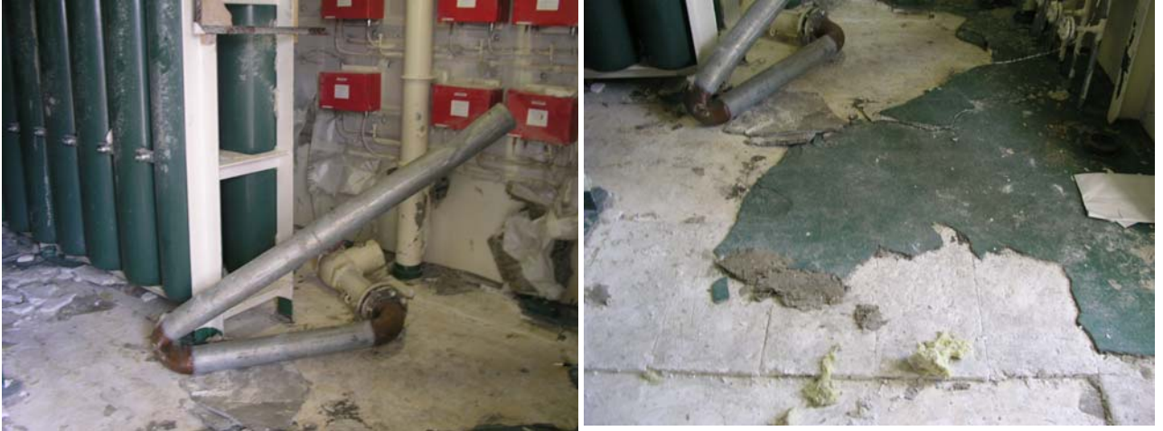
The bended pipe and the damaged floor insulation material after the accident
