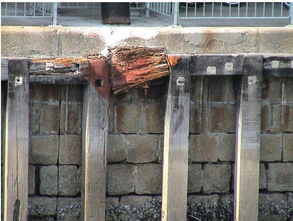
Figure 2 Damage sustained to the seawall
